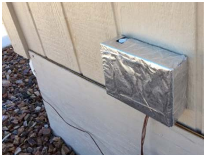
Figure A.4: Installed data logger
